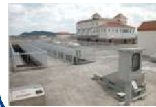
Electrical instrumentation systems for water and sewerage
