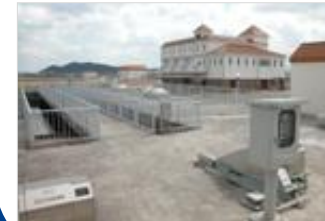
Electrical instrumentation systems for water and sewerage
