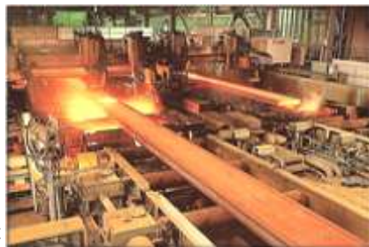
Continuous casting equipment
